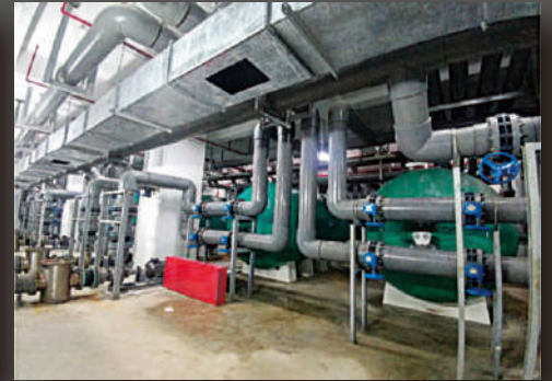
Barangaroo Water Treatment Plant New Wale Wales,Australia
